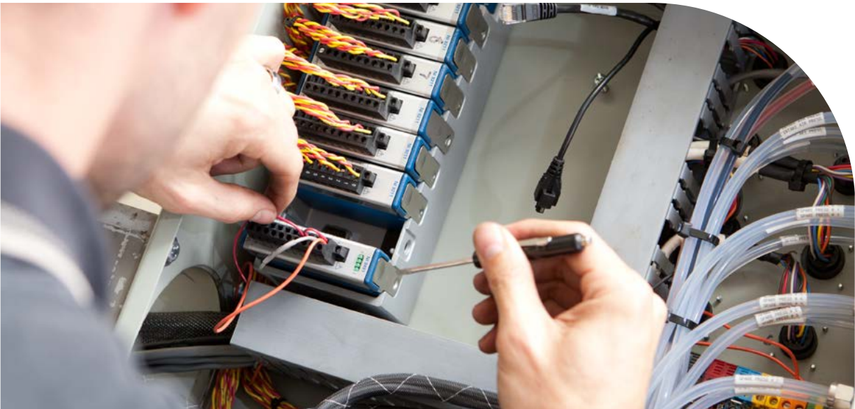
FIG 5 | Standardize on a few module connectors (screw terminals shown in image above) for efficient system assembly and support.
